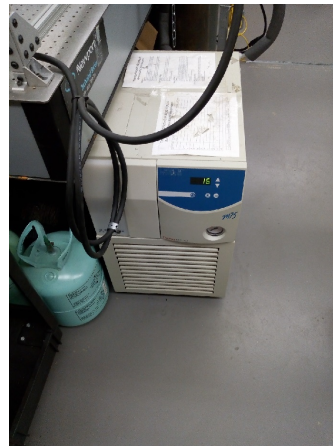
(b) Air chiller
