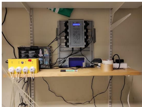
Figure 14: IKS pH control system
