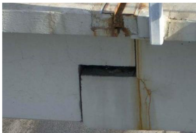
Figure 1.2: Example of a dapped-end connection with durability problems [17]
