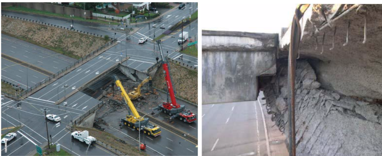
Figure 2.3: Collapse of the Concorde bridge in Quebec, Canada in 2006 [18]
