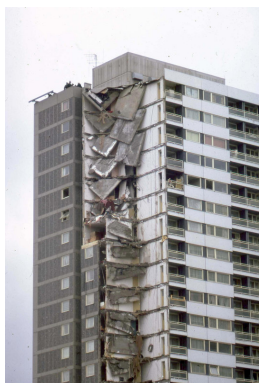
Figure 1.1: Ronan point collapse 1 .
