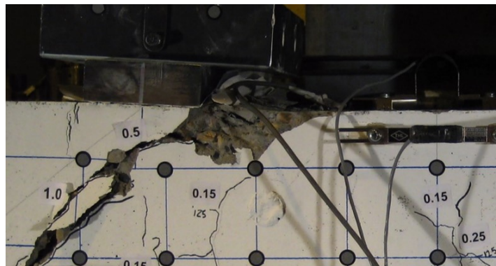
Figure 4.6: Shear-induced flexural crushing in specimen A2N (courtesy by Andermatt and Lubell, University of Alberta)
