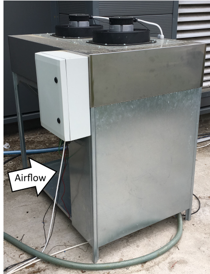
Figure 2.5: Picture of the heat pump
