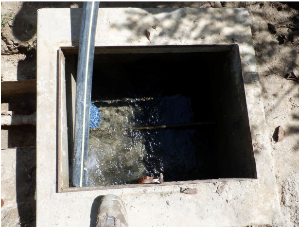
(a) Photo : caisse brise charge.
