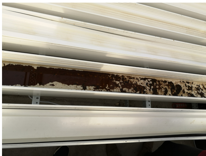
Figure 3.21: Solid residues deposited on the P65C gully.
