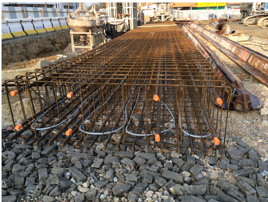
Figure 3.8 – Photo of the pipe cages used in the slurry walls [personal communication]
