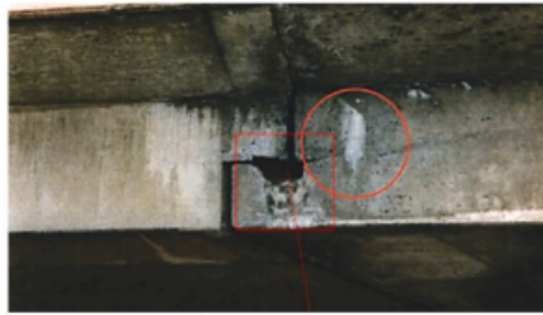
Figure 1.2: Deteriorated dapped-end connection [30]
