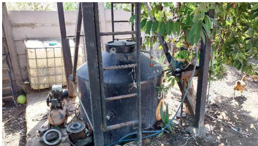
Figure 62: Water tank storage with motorized pump for individual consumption (Photos: H. LE VASLOT)
