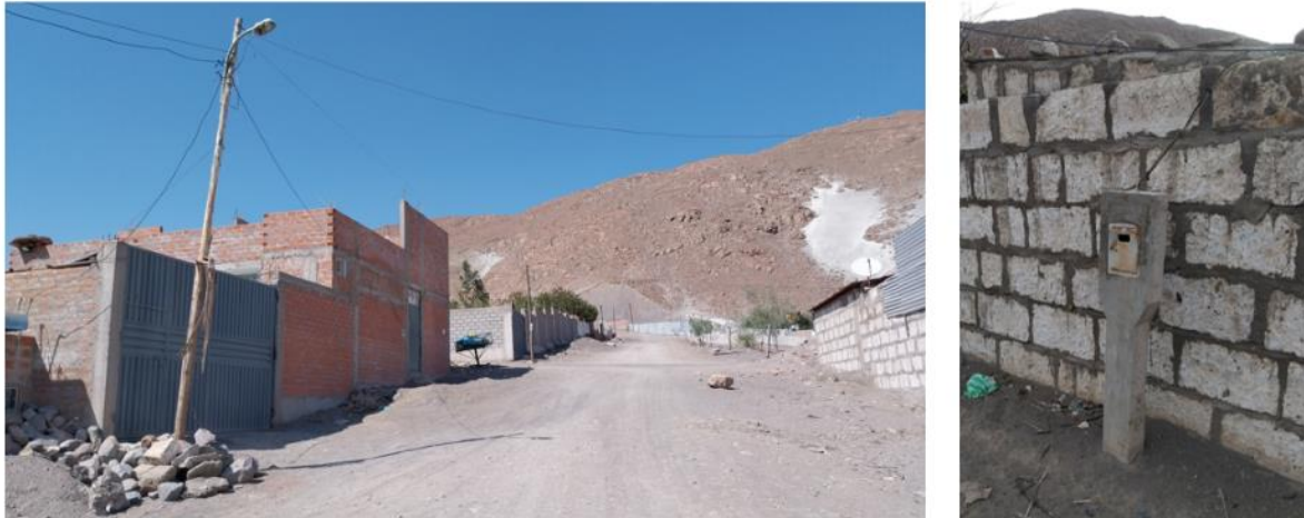
Figure 56: Public lighting network and electrical consumption meter in Virgen del Rosario settlement (Photos: H. LE VASLOT)
