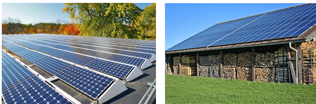
Figure 3.6: (Left) Solar panel installation on a flat roof, (Right) Solar panel installation on an inclined roof
