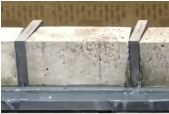
(a) Photo of water leaks
