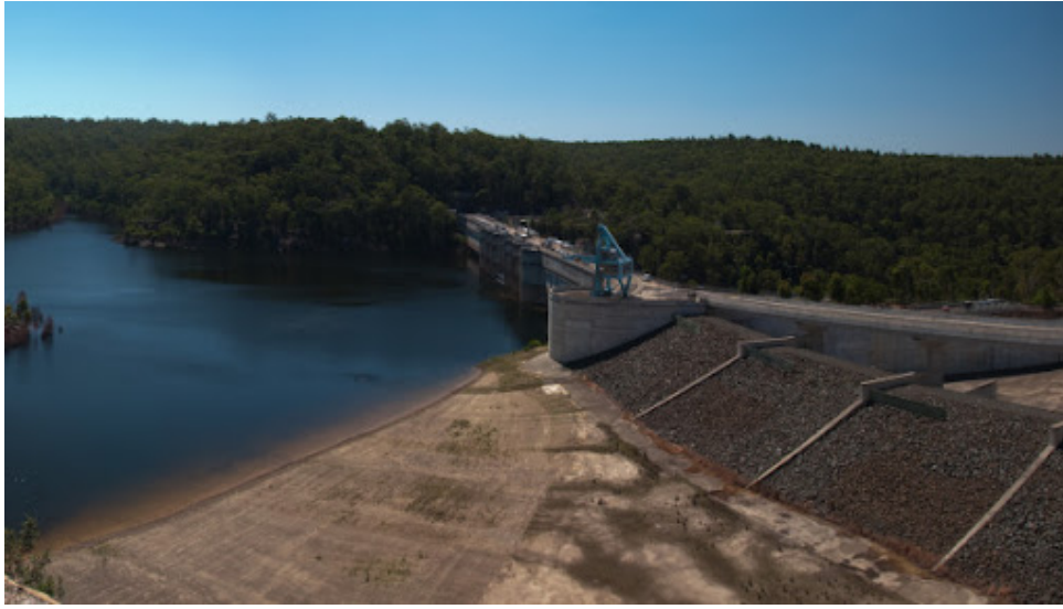
(a) Photo of earth fuse plugs at the Warragamba Dam in Australia (from Reid)
