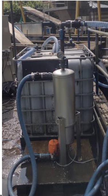
Figure 10 : Photo de l'hydrocyclone
