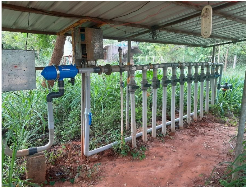
Figure 7: Manual valves for drip irrigation.
