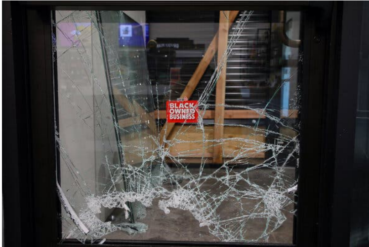
A door broken in a robbery awaiting repair at Blunts and Moore.
