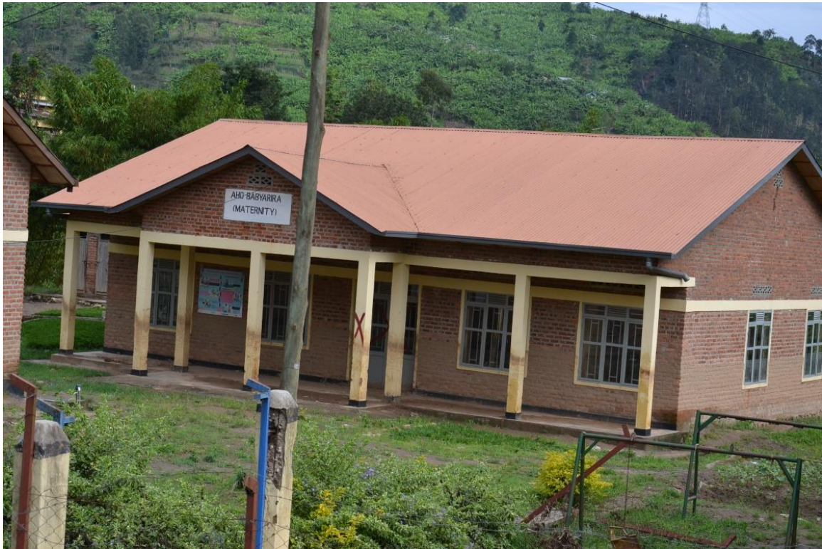
Figure 9. Picture of a maternity hospital affected by the May 2023 floods in Mukungwa watershed marked with a cross meaning that it will be expropriated. Note the mark left by the water, indicating the height reached by the flood (Picture by Victor De Clerck, 2023).
