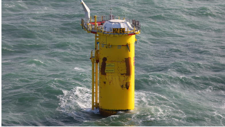
Figure 2: Damaged wind turbine foundation after collision; Source : Buitendijk (2022)
