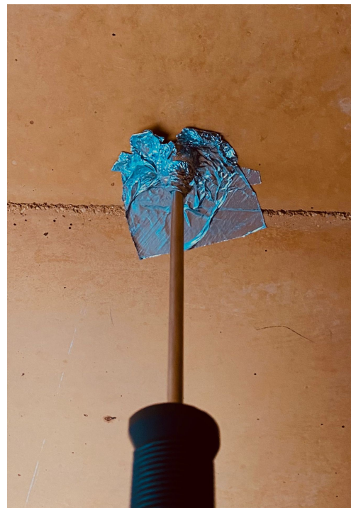
(b) Type-K contact probe installation.
