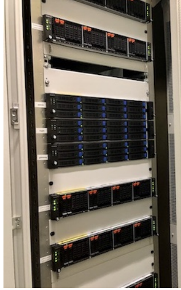
Figure 4.13: View of the physical NIC5 supercomputer racks housed at the University of Liège.
