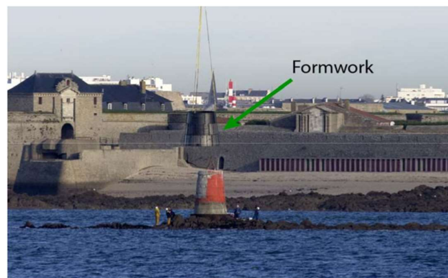
Figure 10 The formwork being placed on the small island, around the tower (Denarié et al. 2013)
