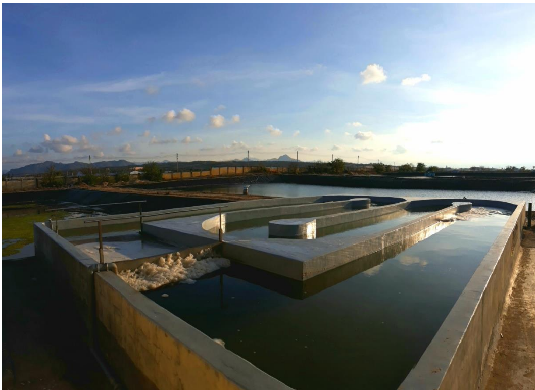
Figure 1 – High Rate Algal Pond pilot installed in Vietnam
