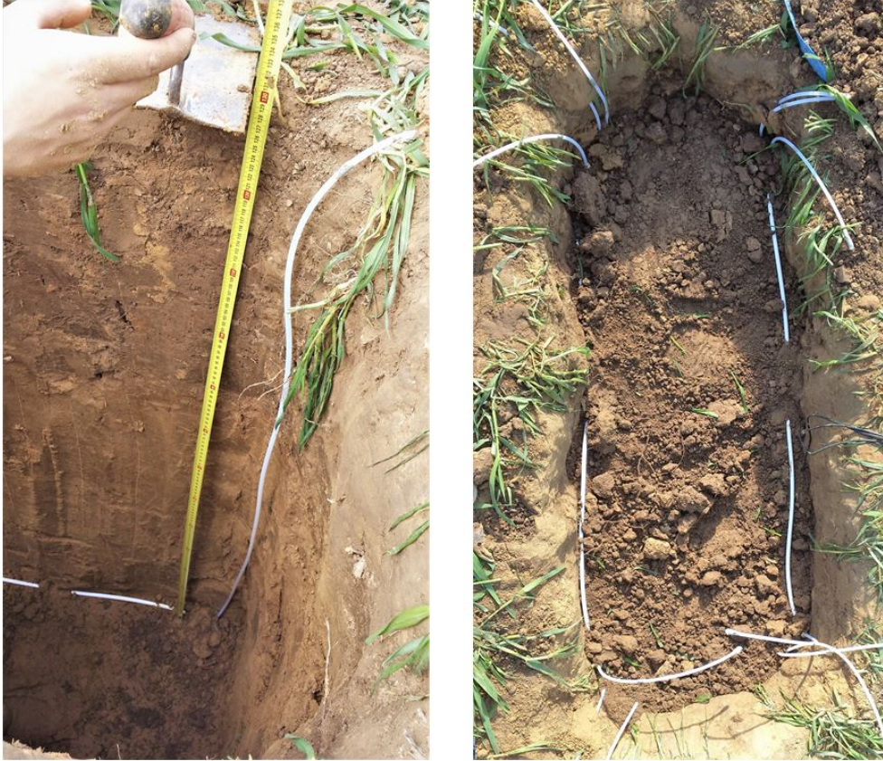
Figure 32: Pictures of the tubing installation. Left picture shows the tubes installed 1.3 m deep while the right picture shows the installation at 0.2 m.
