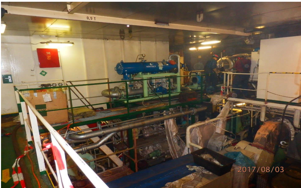
Figure 60: Engine Room of M.V. Main Highway [22]
