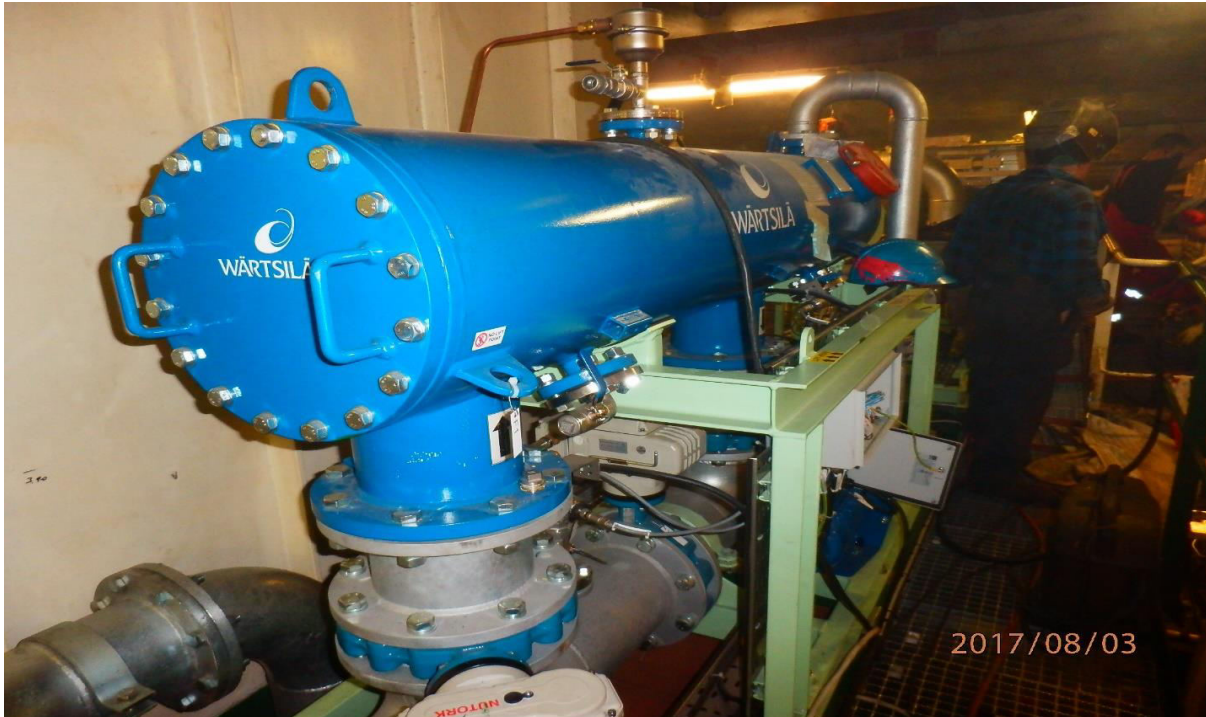
Figure 59: Installation onboard M.V. Main Highway[22]
