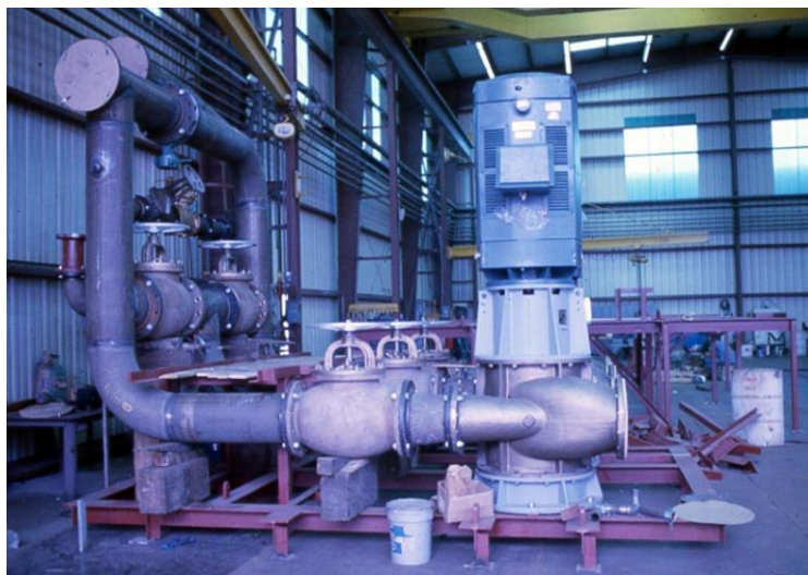
Figure 7. On-unit outfitting package. Pump-set for sea water system (source: http://i0.wp.com/lou.chirillo.com/wp-content/uploads/2014/06/AVON02c.jpg )
