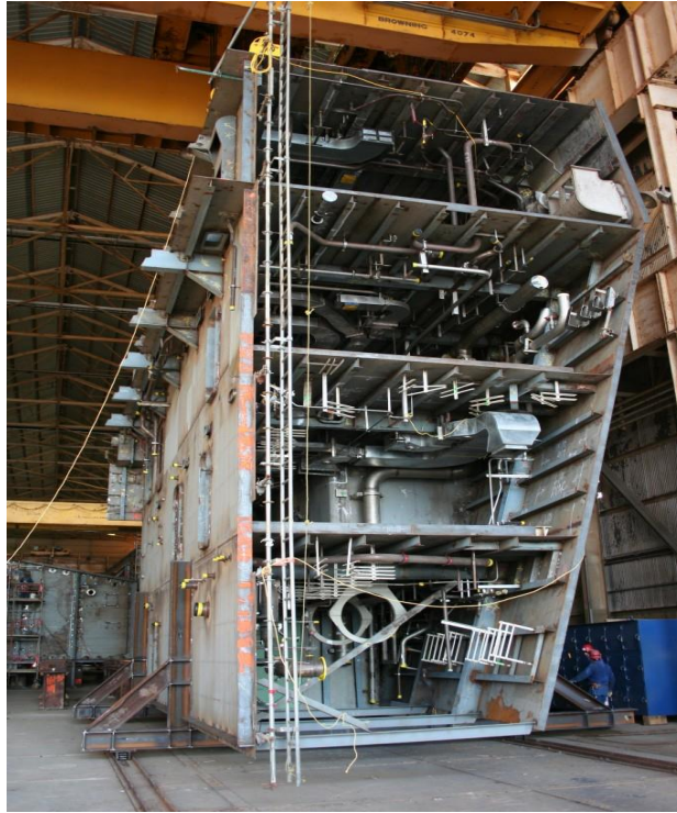
Figure 44. Outfitting on-block assembly (right-side block). Includes pipelines, cable trays, ducting for HVAC system. (source: http://www.worldmarine.com )
