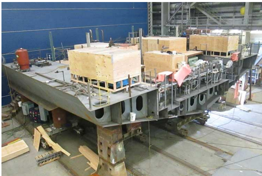
Figure 43. Outfitting on-block assembly (right-side). Includes pipelines, main machinery protected with wooden boxes (gen-sets) and auxiliary machinery. (source: http://dot.alaska.gov/amhs/alaska_class/ )
