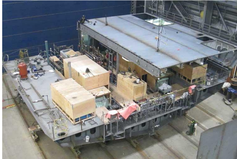
Figure 48. Main machinery protected with wooden boxes, during the installation of another structural assembly above (source: http://dot.alaska.gov/amhs/alaska_class/ ).
