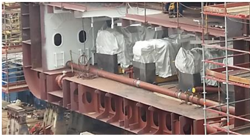
Figure 46. Gen-sets installed on-block stage. (source: fieldwork during internship at CRIST shipyard).
