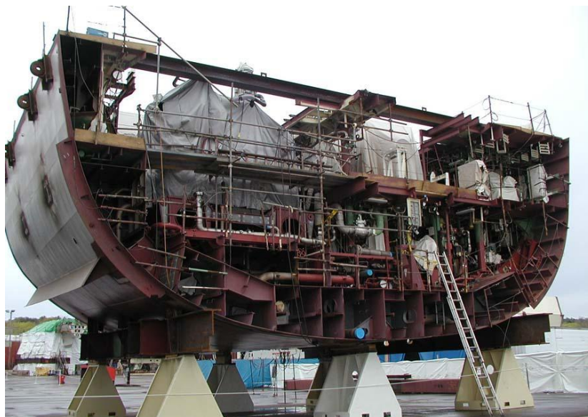
Figure 20. Main Engine Room #2 of DDG 90. This unit contains the complete main machinery (two LM2500 gas turbines and their reduction gear) and generator #2. Total weight approximately 480 tons. (source: https://www.hazegray.org )
