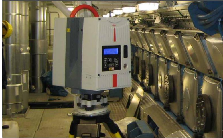
Figure 51. Leica Geosystems High-Definition Surveying (HDS) laser system tracking ship engine room in construction.
