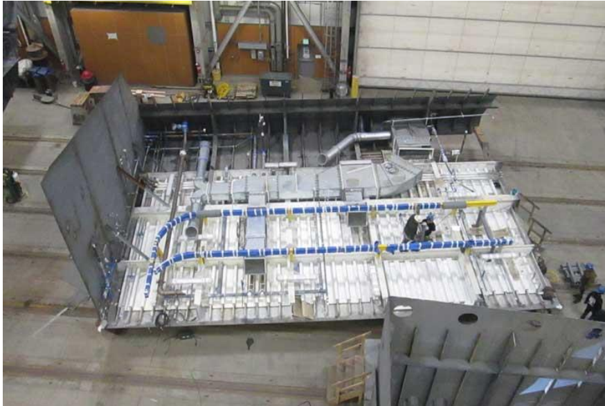
Figure 42. Outfitting on structural assembly unit (upside-down). Includes pipelines, ducts for HVAC system, cable trays. (source: http://dot.alaska.gov/amhs/alaska_class/ )
