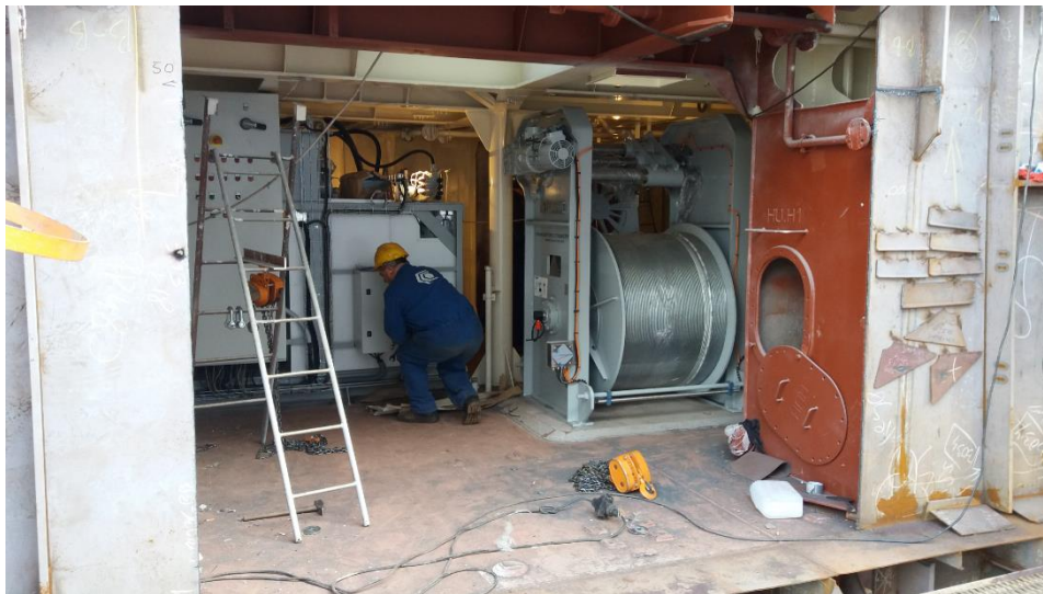
Figure 45. On-block outfitting. Insertion and installation of auxiliary machinery, in this case a dynamic pull system. (source: fieldwork during internship at CRIST shipyard)
