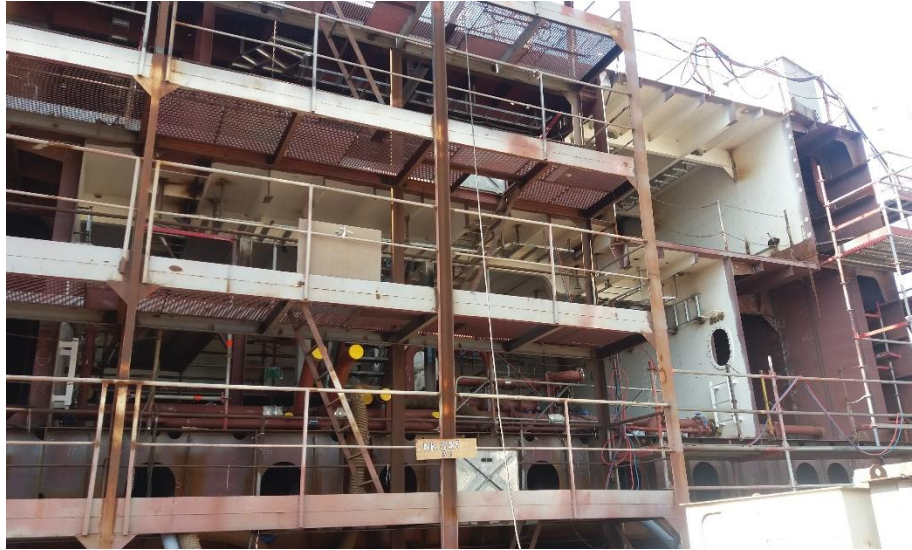
Figure 50. High quality and design scaffoldings allow carried outfitting activities safer and faster. (source: fieldwork during internship at CRIST shipyard)
