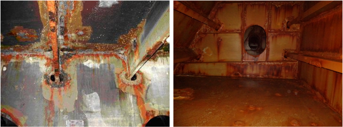
Figure 1: Corrosion Affected Areas
