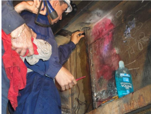
Figure 23 - Welding on the side shell checked with dye penetrant and ultrasonic equipment to detect flaws
