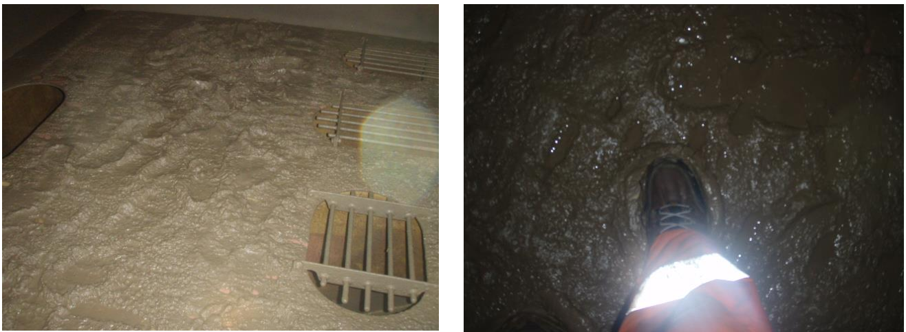
Figure 21 - Typical slippery mud inside ballast tanks
