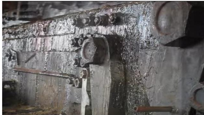
Fig.26. Open Trigger device. It is possible to show the retention structure in the slip truck [23]
