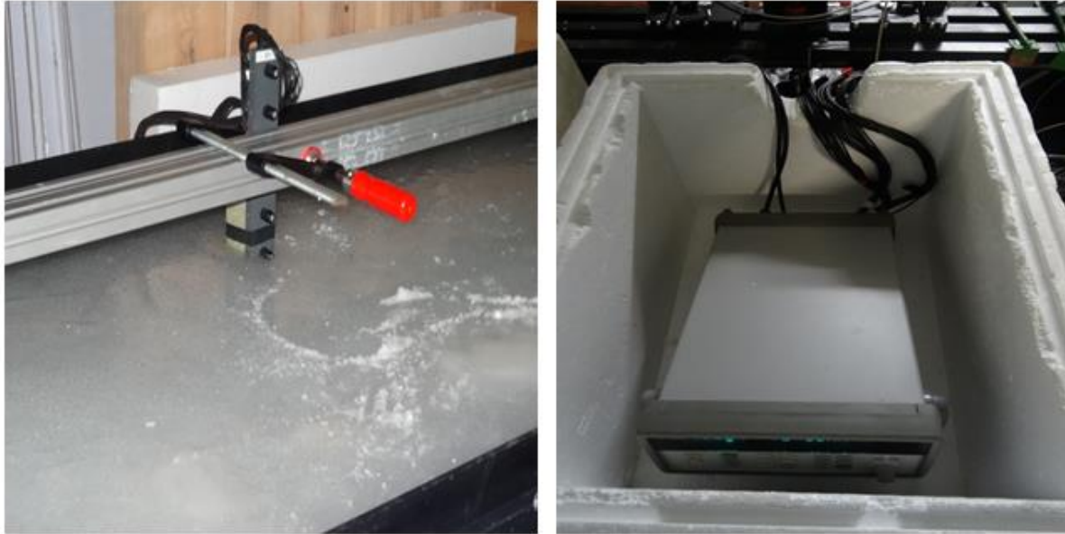
Figure 24 Temperature Sensors Installation
