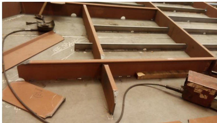
Figure 3.97 Poor junctions between stiffeners
