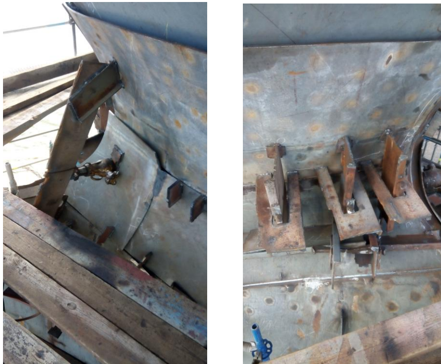
Figure 3.99 Not achieving proper curvature of steel plate
