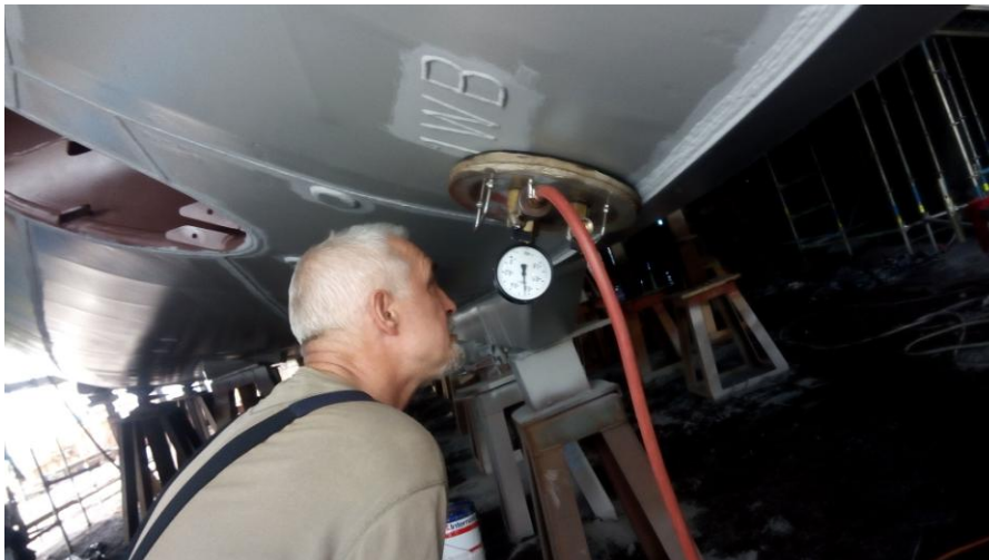
Figure 3.77 Leakage test for holes
