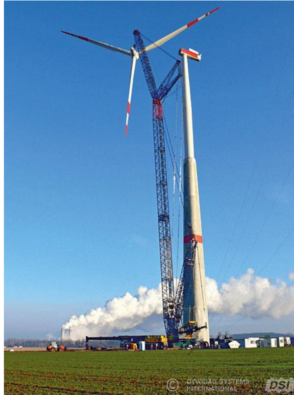
Figure 23: Assembly process for hybrid tower (“Prefabricated DYWIDAG Tendons Secure Innovative ATS Hybrid Wind Tower - DYWIDAG-Systems International” n.d.)
