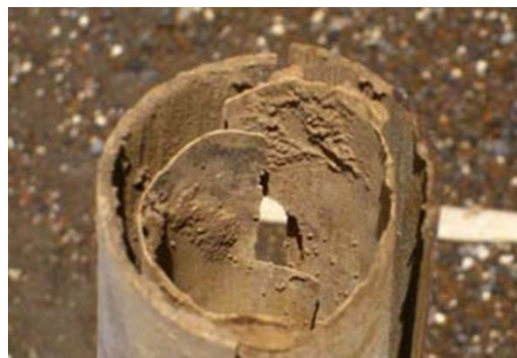
FIGURE 23 - TERMITE DAMAGE ON A BAMBOO POLE, ASALI BALI
